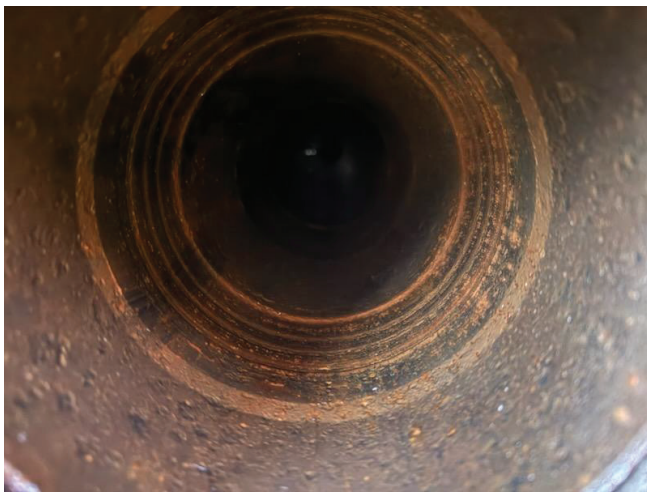
Figure 1: Corrosion on the interior of the temporary well's pump chamber. This is not a suitably inert environment for samples where metal and nitrate concentrations are of interest.
