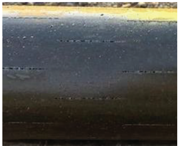
Figure 2: Custom machined 'screen slots' that provide much less surface area for water entry than a typical screen. Remaining area likely reduced to ~50% of that by sand particles becoming lodged against the slot sidewalls. This likely contributed significantly to the excessive drawdowns observed in the casing during pumping.
